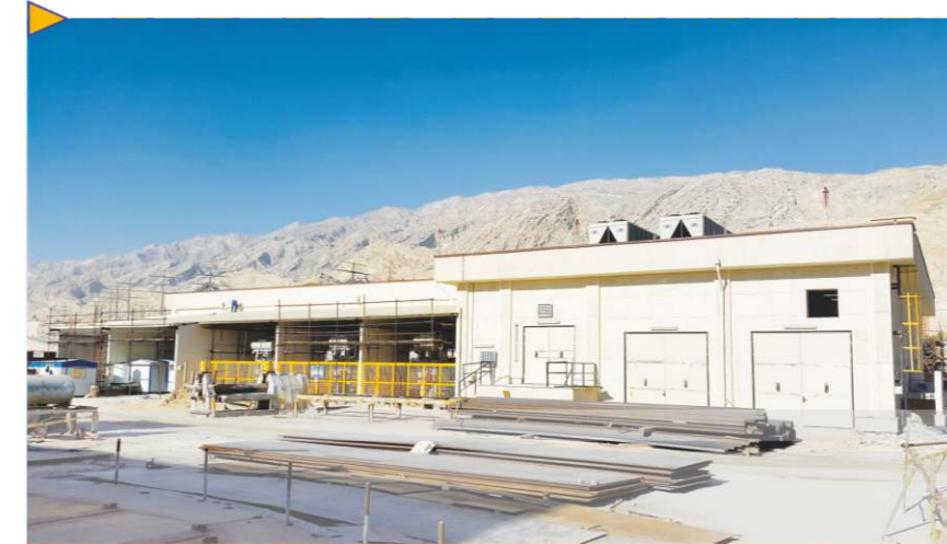
Civil Works, Industrial Civil & Underground Pipeline of Sweetening Unit of Boushehr Petrochemical Complex in Asaluyeh
