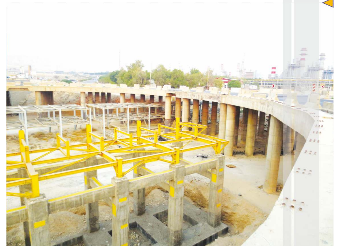
Civil Works & Concrete Structures Construction of Morvarid & Kavian Petrochemical Complexes in K2 Route in Asaluyeh ( Connecting Bridge of Phase 1 & 2 )
