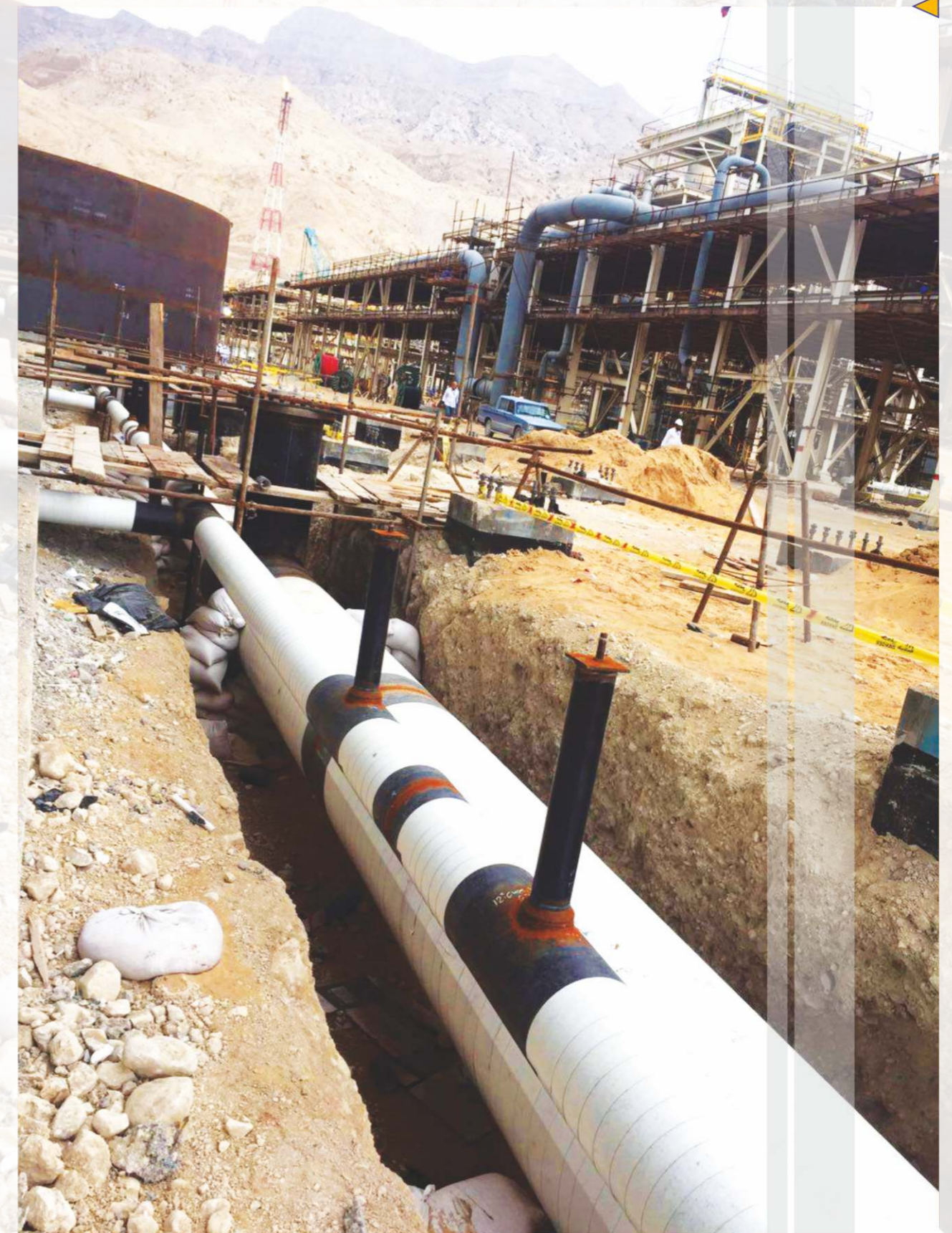
Inlet & Outlet Pipes Implementation of Boushehr Petrochemical Complex Cooling Towers in Asaluyeh (Site 3)
