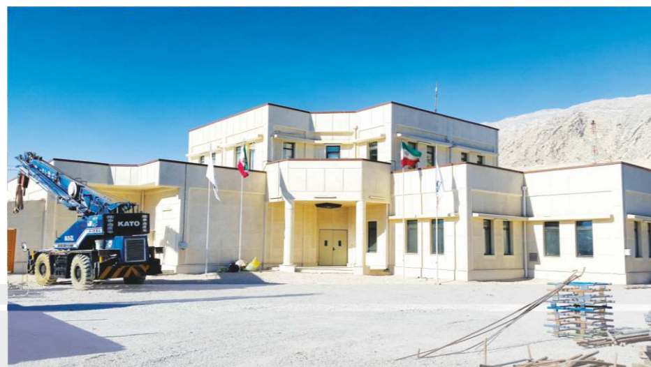
Civil Works, Industrial Civil & Underground Pipeline of Sweetening Unit of Boushehr Petrochemical Complex in Asaluyeh
