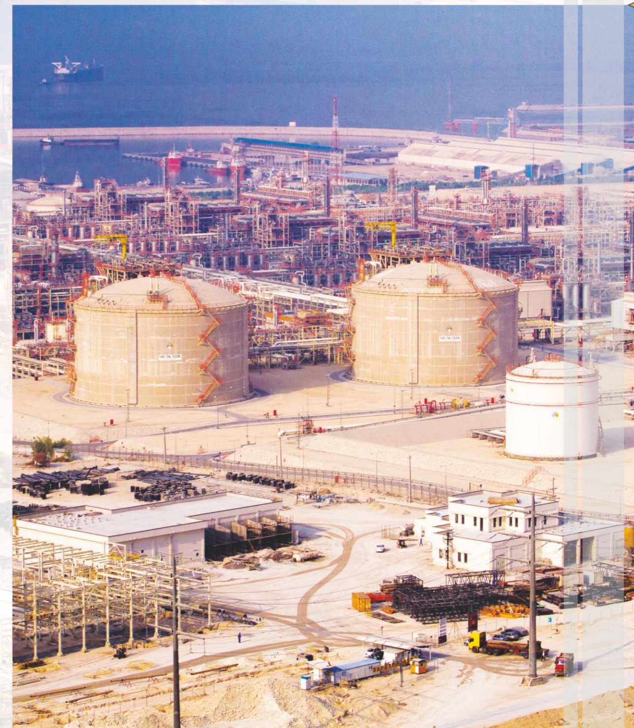
Civil Works, Industrial Civil & Underground Pipeline of Sweetening Unit of Boushehr Petrochemical Complex in Asaluyeh
