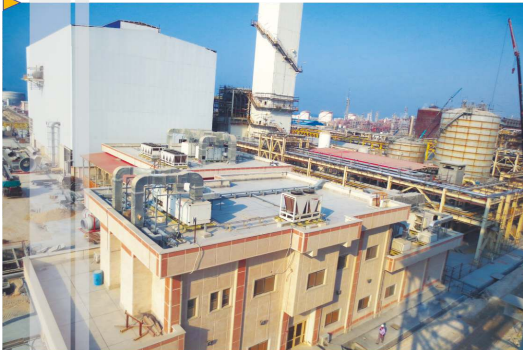
Industrial Civil Works, Building & Underground Pipelines of Air Unit Project (ASU) of Boushehr Petrochemical Complex in Asaluyeh
