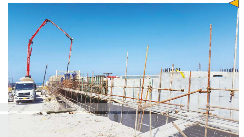
Construction of West Wall of Site 2 of Boushehr Petrochemical Complex in Asaluyeh
