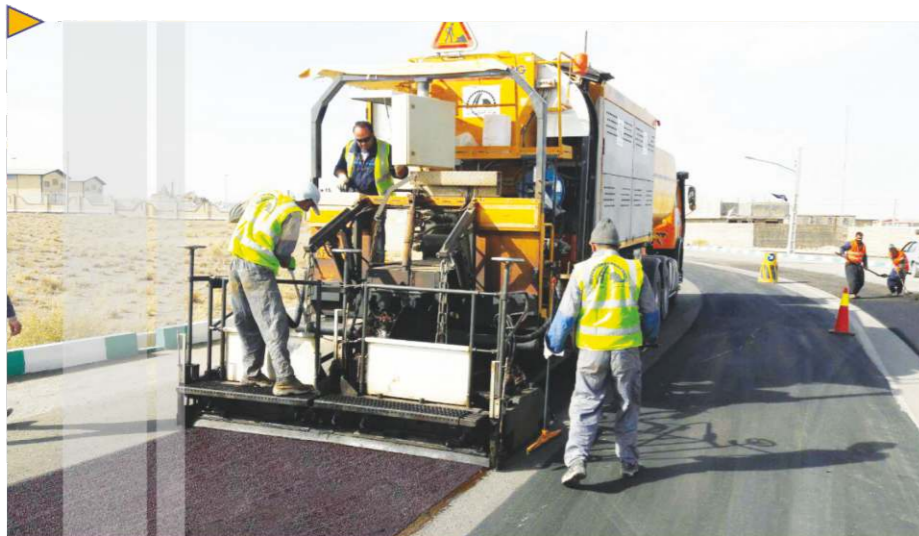
Protective Cape Seal Asphalt Pavement Containing One Layer of Chip Seal & Two Layers of Microsurfacing in Salafchegan-Delijan
