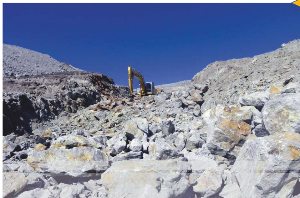
Construction of Access Road for Water Conveyance from Hajjiarchai Dam to Songoon Lead Complex
