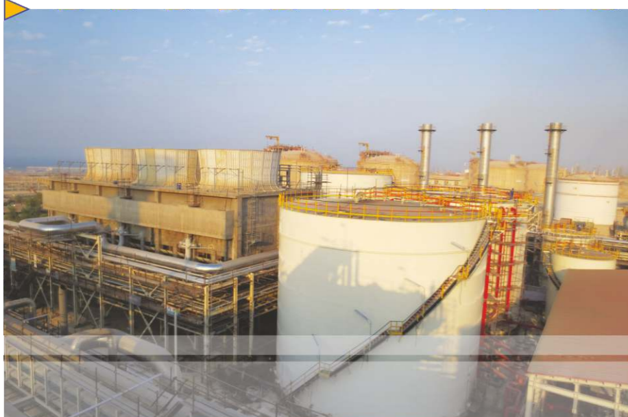
Civil Works & Concrete Structures Construction of Cooling Tower of Boushehr Petrochemical Complex in Asaluyeh (Site 3)
