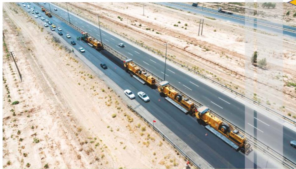
Design, Construction & Rehabilitation of Karaj-Hashtgerd-Abyek Road by Hot In-place Recycle & Polymer Modified Asphalt Overlay Method
